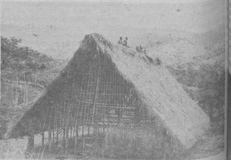
This picture shows the top almost complete and the grass being applied to one of the gable ends.
