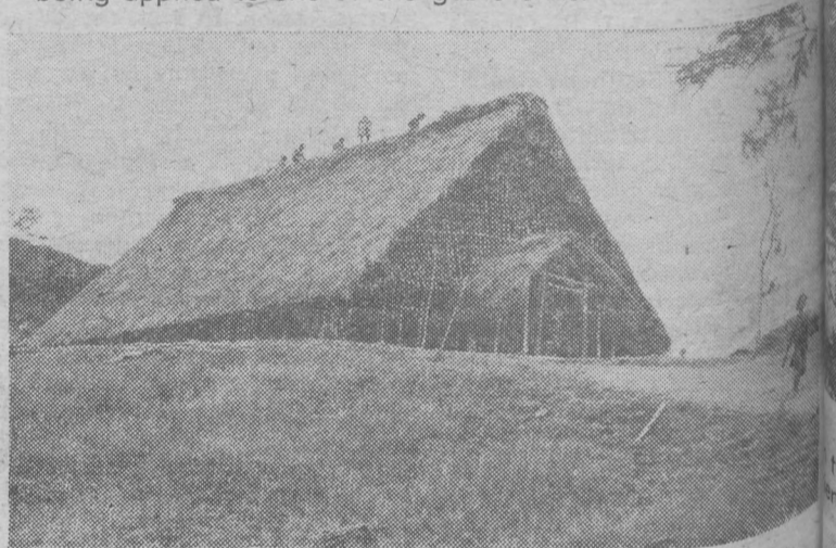
Here the building is nearly complete insofar as the superstructure and the top are concerned. A few days later we started having services in the building.
